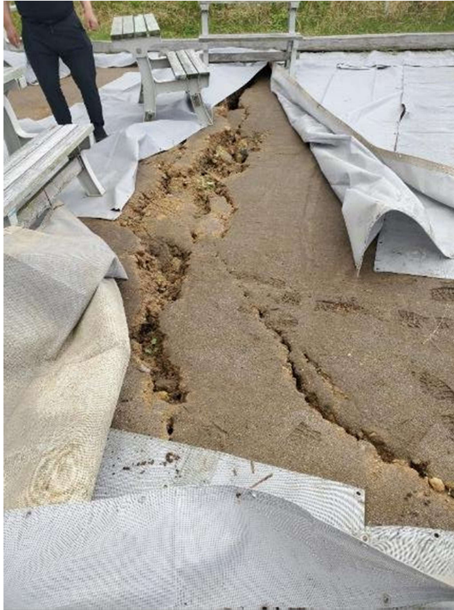
Cracks in salt farm
